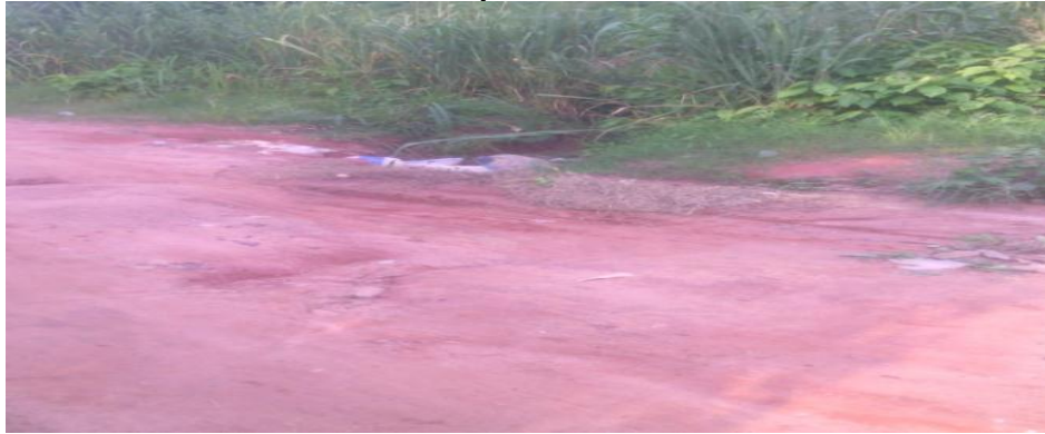
Plate 1: Erosion at site A
