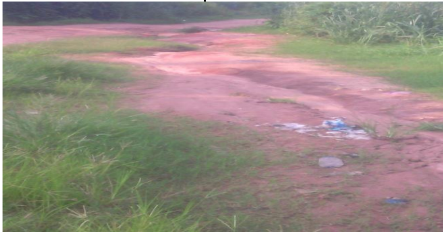
Plate 6: Erosion at site F
