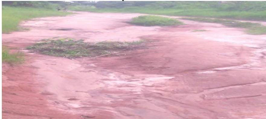
Plate 5: Erosion at site E
