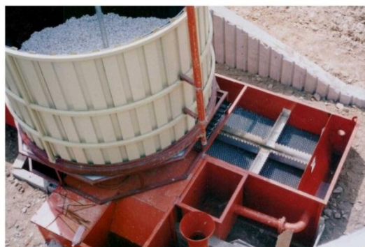
Fig. 1. "Ekogramont" - biological wastewater treatment plant
